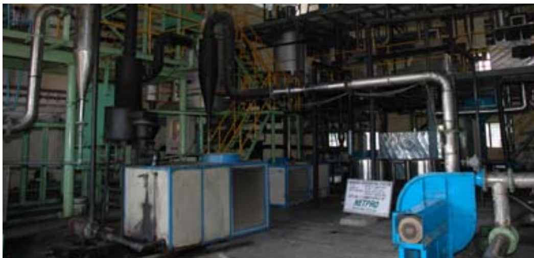
Biomass gasification system
