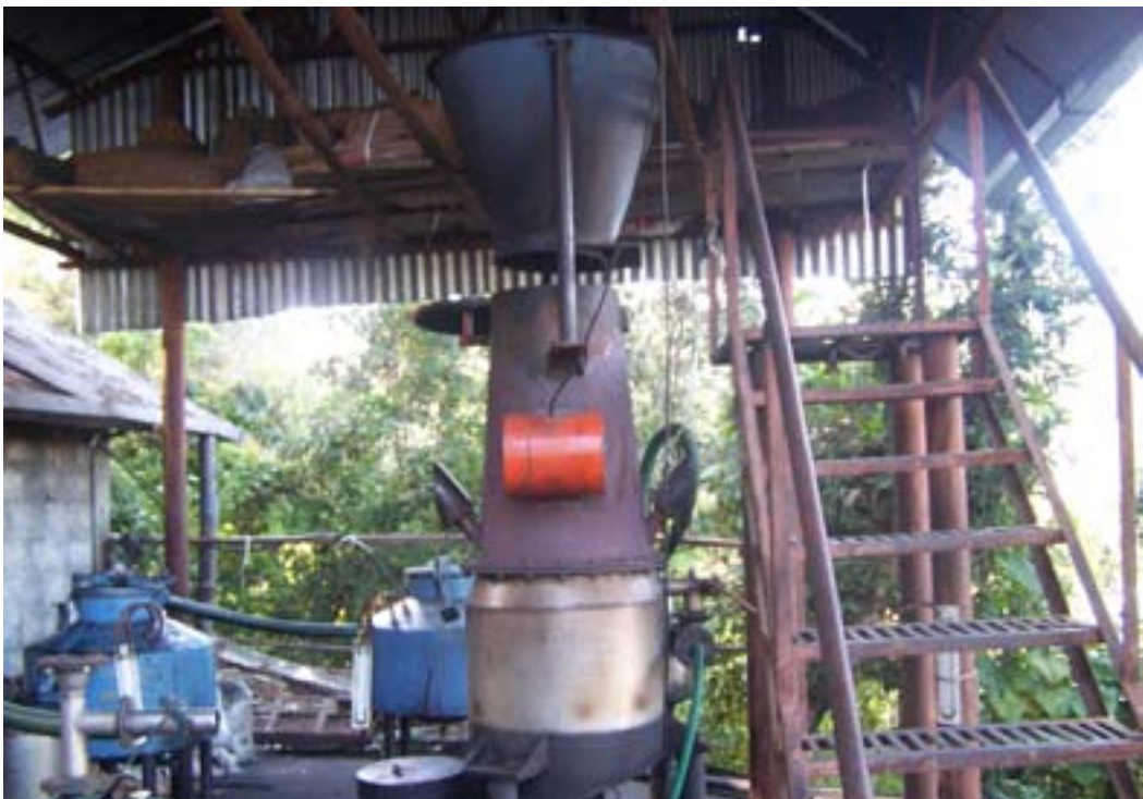
Equipment for gasification of pine needles
