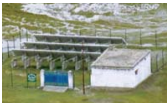
Solar photovoltaic power plant at Juldo
