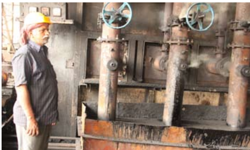
Front view of the energy-efficient re-heating furnace at Pulkit Steel Rolling Mills, Puducherry
