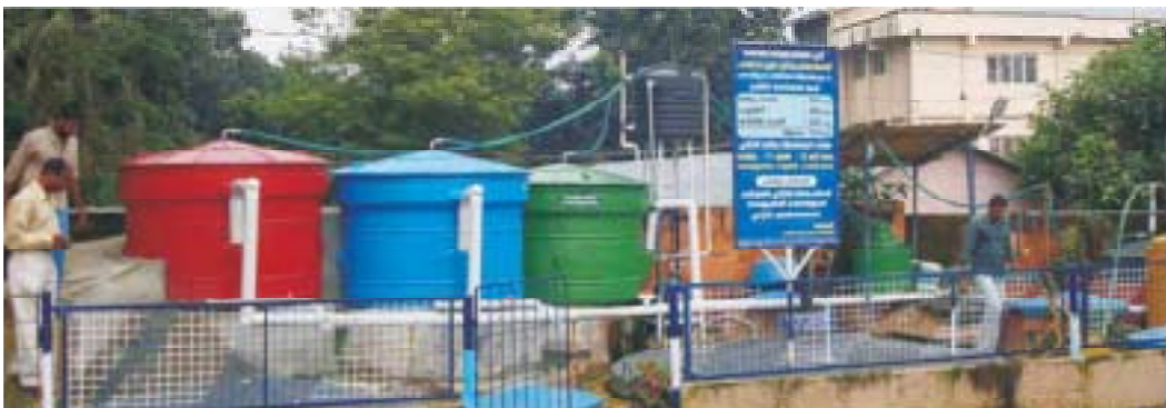
Biogas unit in Pathanapuram
