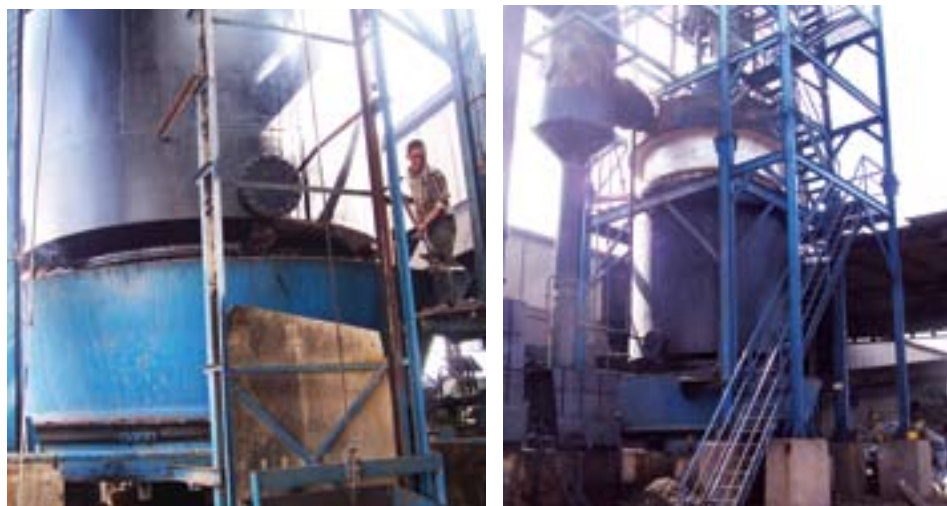
Biomass-based producer gas plant at Pulkit Steel Rolling Mills, Puducherry
