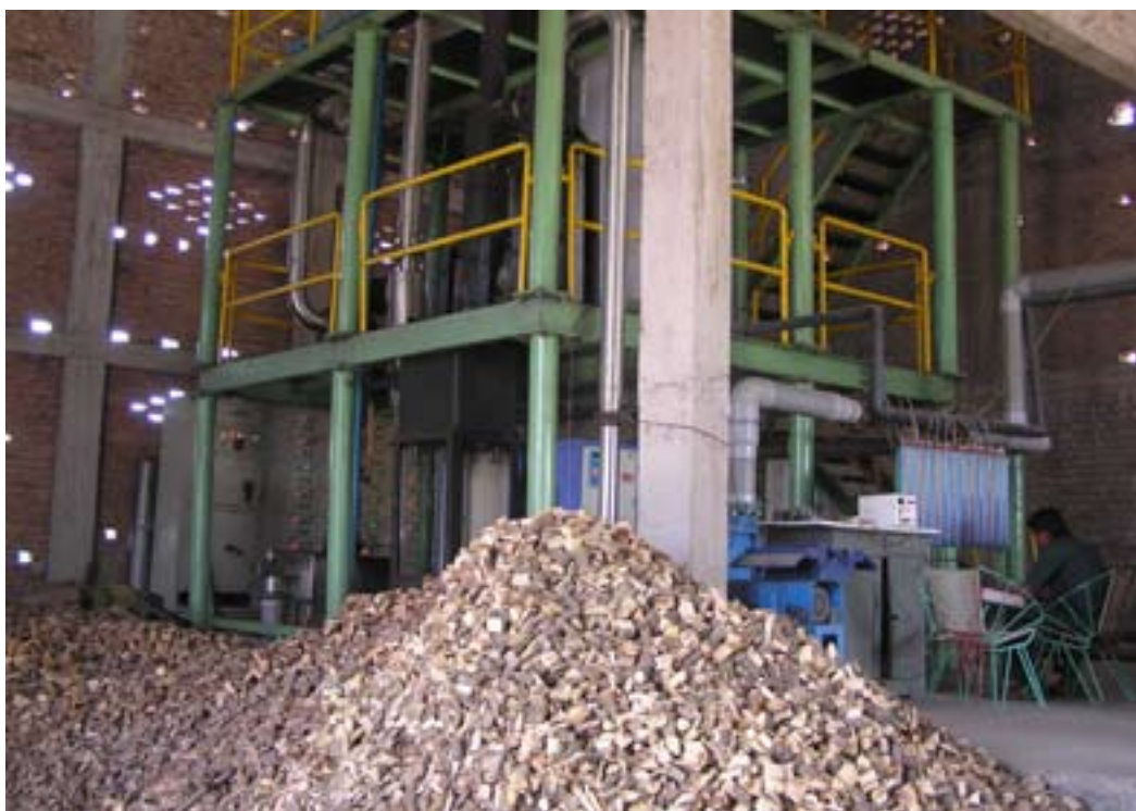
Biomass-based power plant
